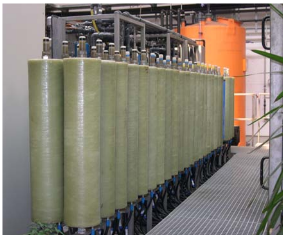
Landfill Wehrden, County of Höxter – Leachate Treatment with Reverse Osmosis
