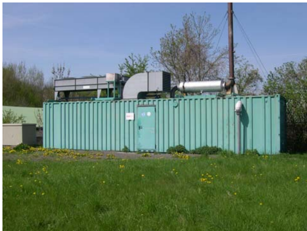
Container Unit for a CHP
